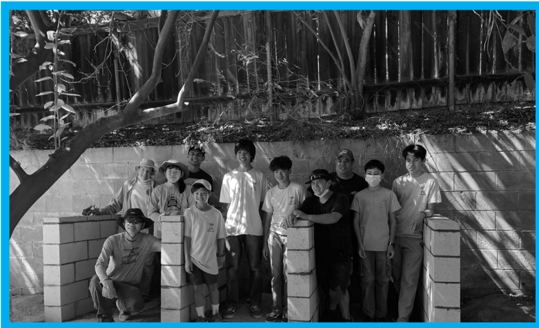
Eagle Scout Bruce Wiles and volunteers from Scout Troop 509 spent a long weekend constructing a composting enclosure near the Lanterman House garden.
